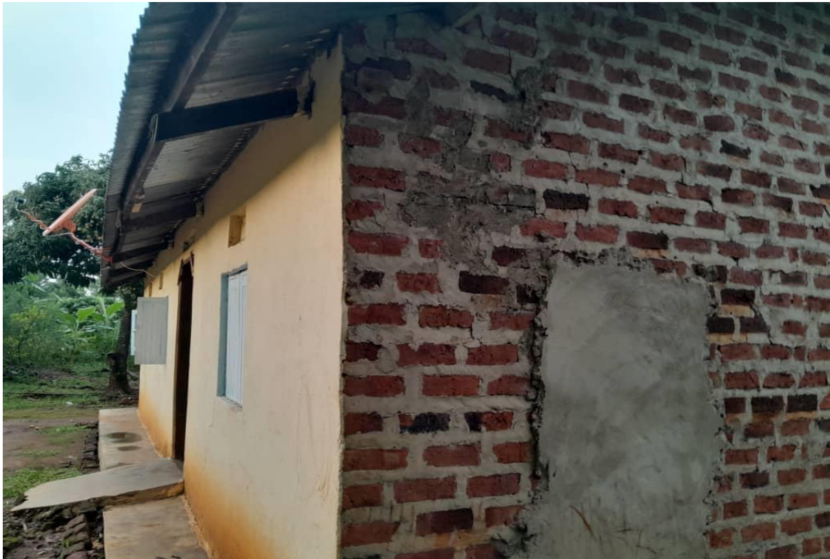
One resident's House cracked by CICO heavy tracks near stone quarrying site.
